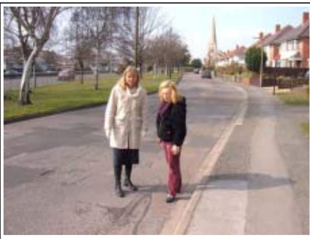
Cllr Virginia Moore and Ceren Davis inspecting the poor road surface on the service road by Millbrook Road . This is on the programme of works to be resurfaced under the £18.5M investment by the Lib Dem administration.
